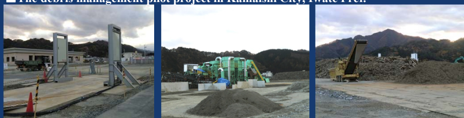
A facility to check radio active contamination A facility to crush debris into small pieces Wooden debris categorized by size
