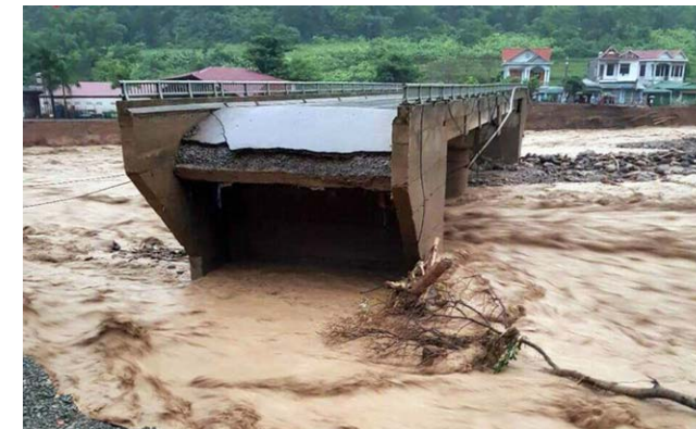
Nặm Păm Bridge in Sơn La was broken by flash flood from 03-06 Aug 2017
