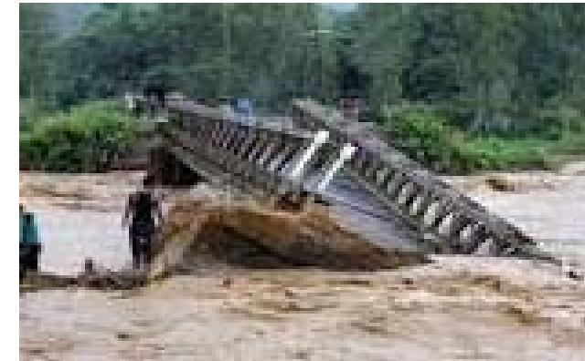
Flash flood, landslide in Lao Cai, 2016
