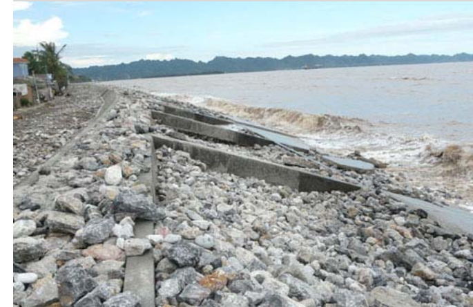
rip-rap revetment with frame was broken by wave
