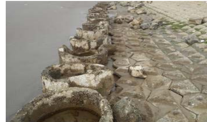
Cement pipes at toe of revetment were broken by erosion
